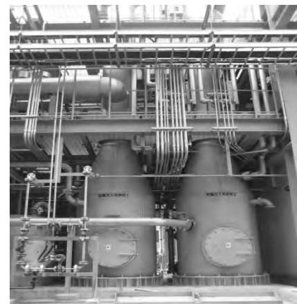
Fig. 4 Gas purification facilities
