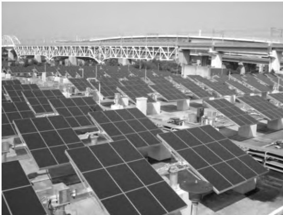
Figure 8. Solar cell generators (single-axis tracking type)
