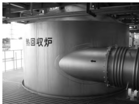
Fig. 5 Heat recovery facilities
