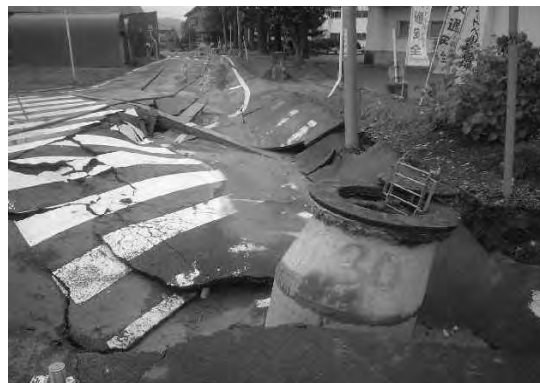
Photo 2: Uplifted manhole (2004 Niigata Chuetsu Earthquake)
