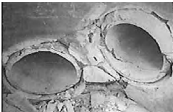
Photo 1: Ruptured connection between manhole and sewer pipes
